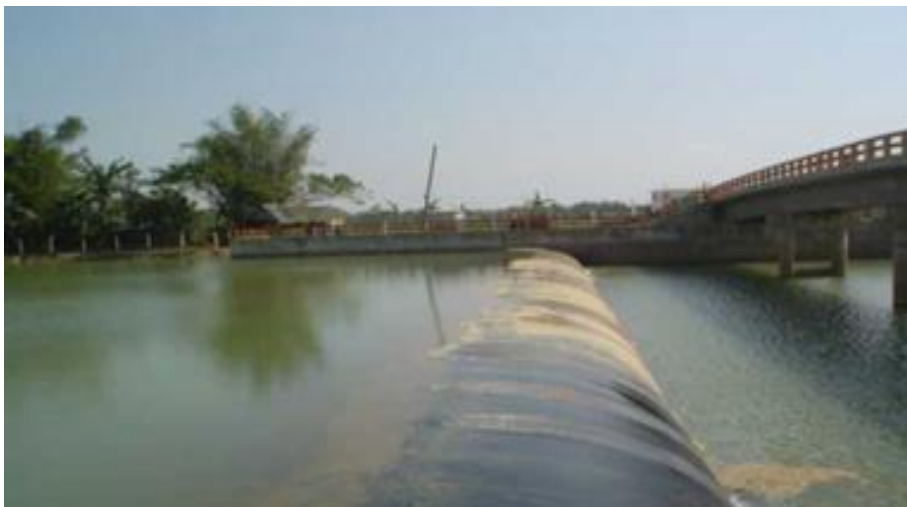
Figure 1. Typical view of Rubber Dam
