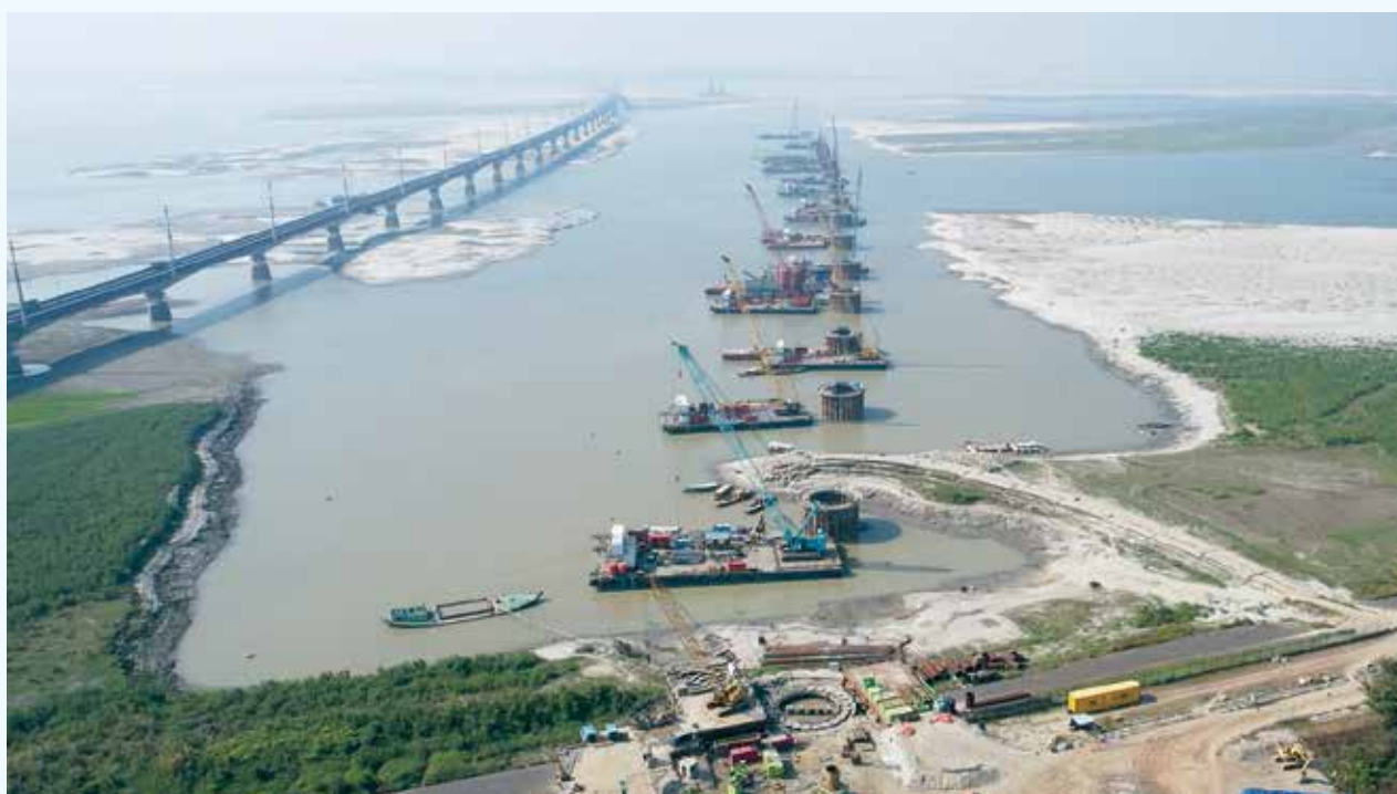
Ongoing Construction of the Bangabandhu Sheikh Mujib Railway Bridge on Jamuna River
