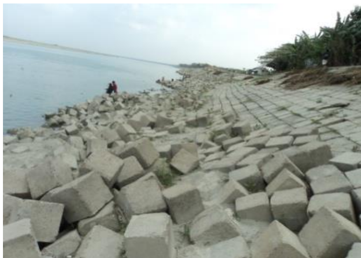
Figure 2.1: Damaged revetment on the right bank of Padma river (d/s of Dholarmore, Tepakhola, Faridpur Sadar, Faridpur)
