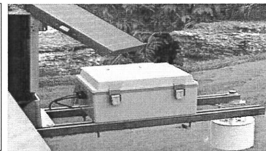
Typical Instillation of AWLG over a Bridge
