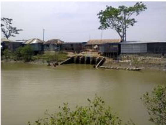
Figure A 2: Damaged Structure at the Mouth of Nolian River
